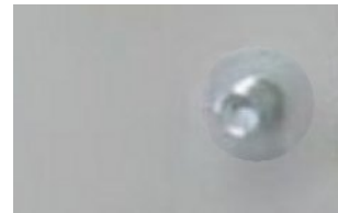
Fig. 24: Unmarked grounding stud
