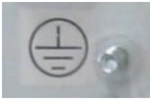
Fig. 23: Grounding stud marked with PE symbol
